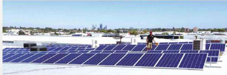
15kw Perth, Australia
